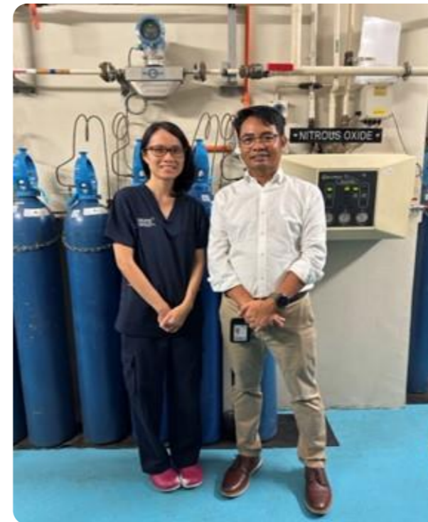
Dr Ang King Sin (left), Consultant, NUH Dept of Anaesthesia and Nay Myo Htet, Snr Engineer, NUH OSS-GFM, leading the N 2 O pipeline shutdown project in NUH
